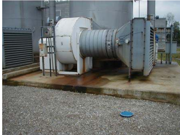
Figure 3 – Example of tower basin and blower.
