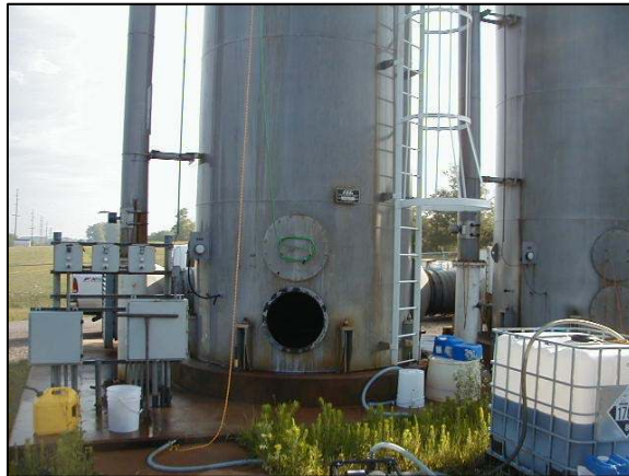
Figure 5 – Example of manway hatch cover.
