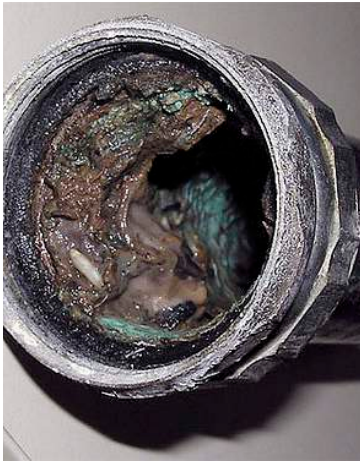
Biofilm coating the sides of a kitchen drainpipe
