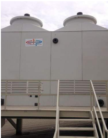
Cooling towers are considered a risk factor for Legionella in building water systems.
