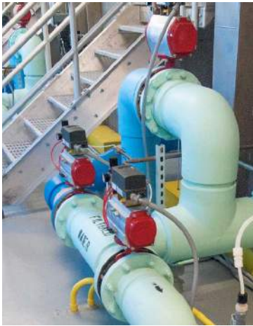
Building water system
